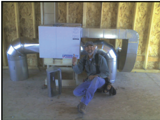
Heat Recovery Ventilation (HRV) Unit
