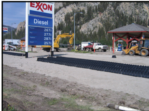
Commercial Septic System Elevated Sand Mound Drainfield
