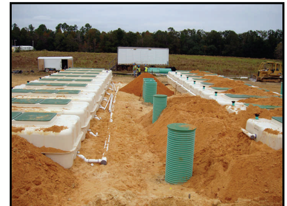
Large Multi-User Advanced Treatment System
