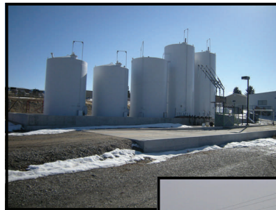
Bulk Fuel Facility w/ Loading Dock
